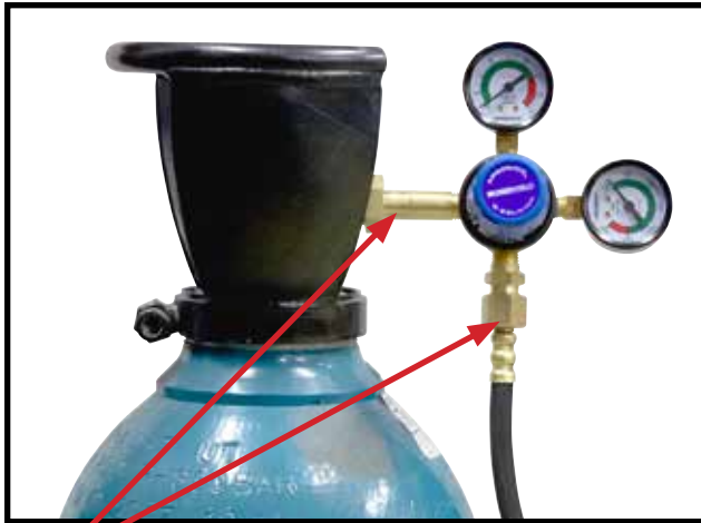
15 Fit gas regulator to the gas bottle and install gas hose from the front of the interconnecting cable to the regulator
