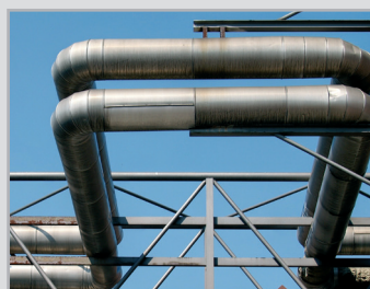
Pipelines subject to pressure
